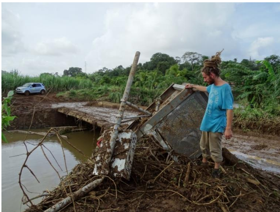
Figure 3 : Destruction de la station GG
