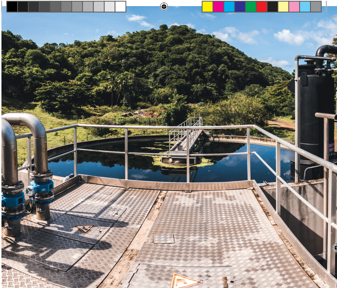
Station du Carbet Bourg – Photos Lucas PELUS ODE
