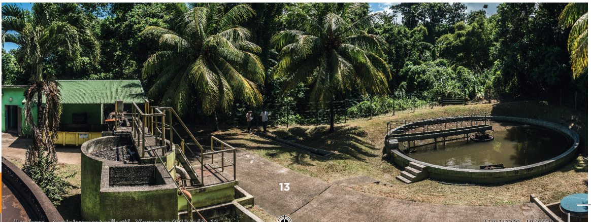
Station d'épuration - Hackaert - Basse-Pointe
